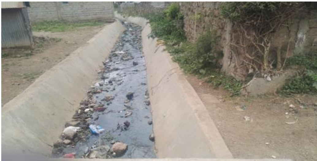
Image 3-13: Polluted Drain in Gataka, Ongata Rongai
